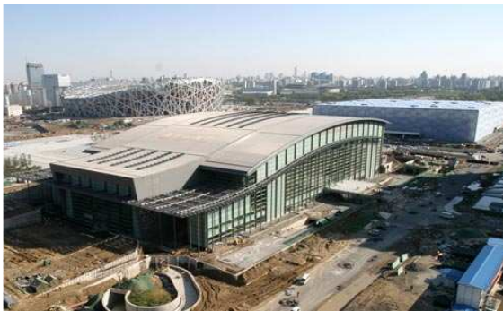
The Olympic Sport Arena in Beijing under construction. View from the outside.
