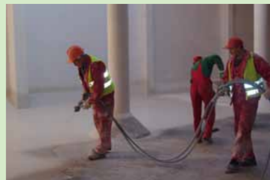
Drinking water tank, Tarnów, Poland
